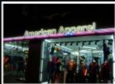
Exposed cold cathode signage
